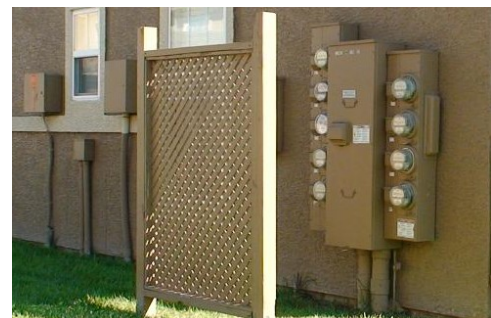
The meters are painted to match the building.
